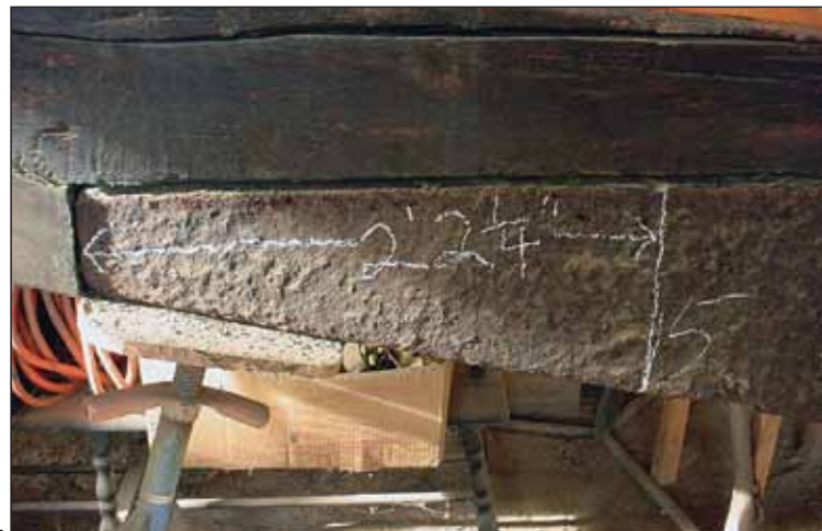
ELF's original lead ballast keel had been taken off during World War I drives for war materiel. The replacement cast-iron keel lasted until Rick Carrion's restoration, when a new lead ballast keel was cast to support a return to her original, large sail plan.
